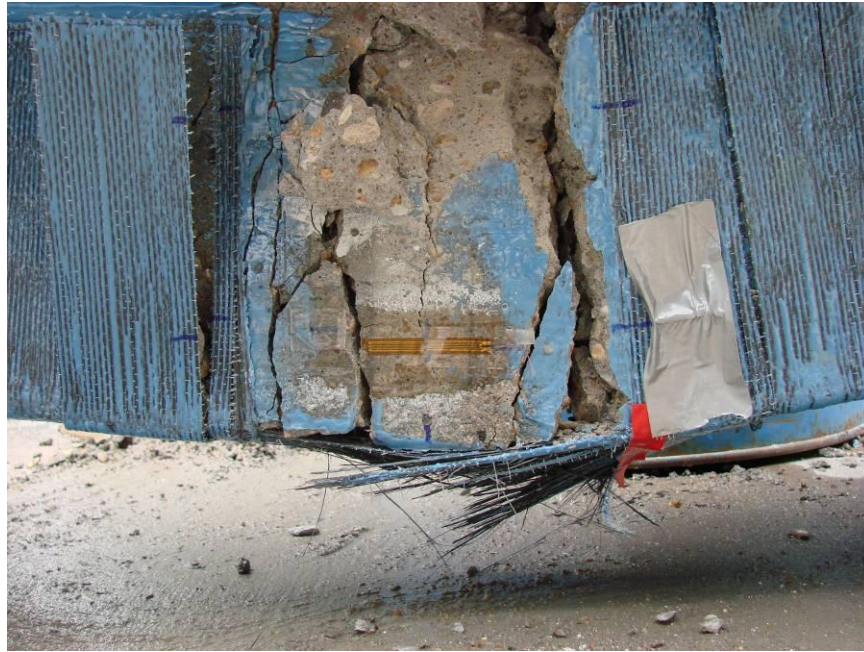
Figure 5.33 Rupture of Flexural CFRP at Mid-Span
