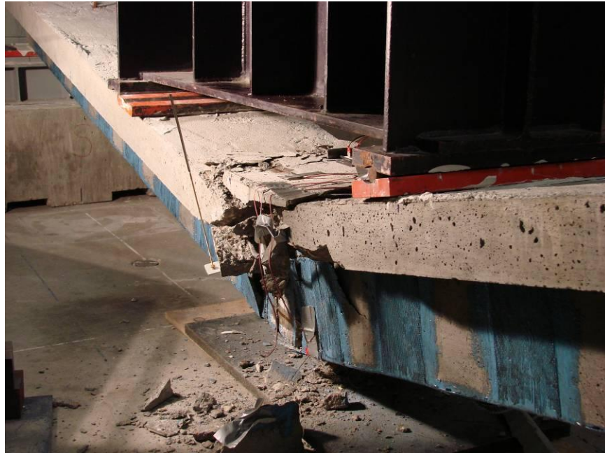
Figure 5.32 Failure of Beam T3 by Rupture of Flexural CFRP
