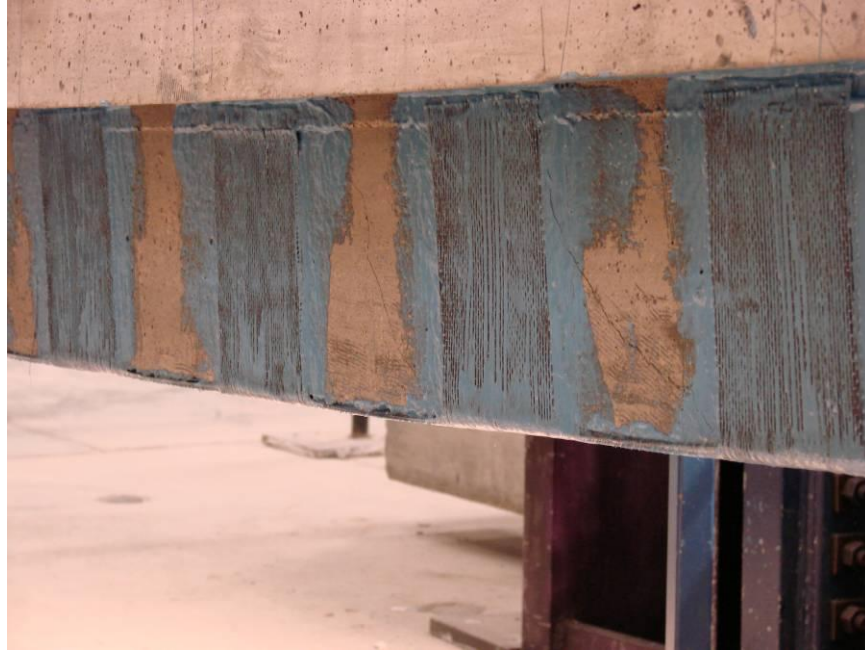
Figure 5.31 Debonding of Flexural CFRP between the U-Wraps
