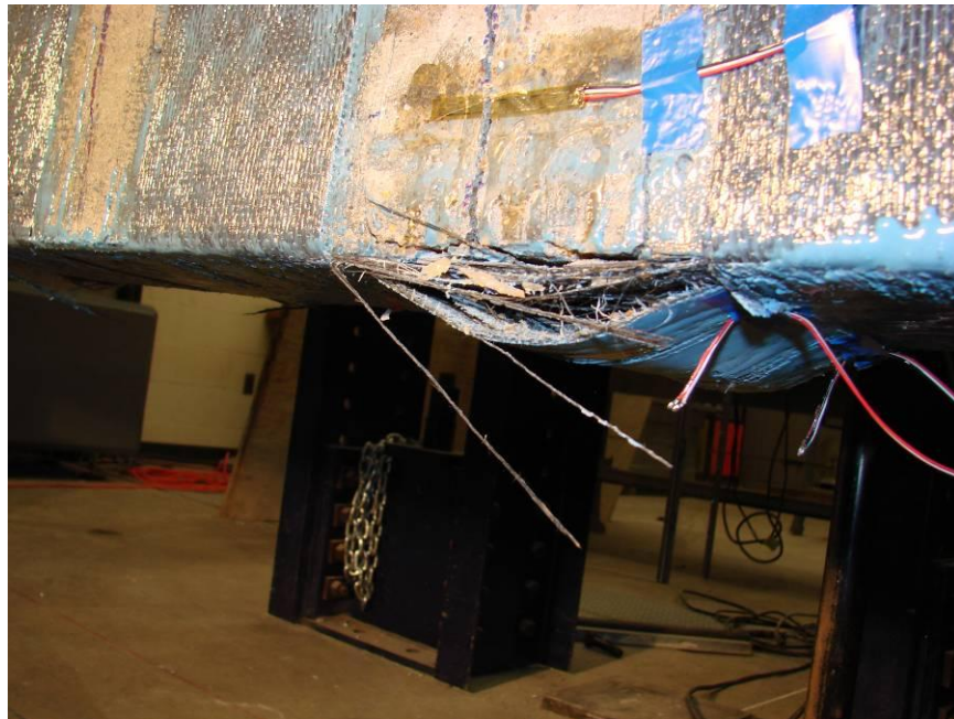
Figure 5.12 Rupture of Flexural CFRP on Beam R3
