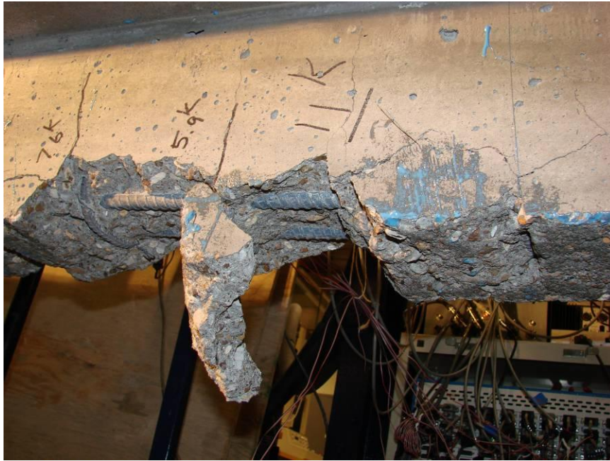
Figure 5.28 Failure of Flexural CFRP by Separation of Concrete Cover
